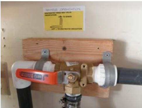
Figure 2. A laundry to landscape graywater system 3-way valve separates water destined for the sewer from water used to irrigate landscape plants (source: http://centralcoastgreywater.org/ ).
